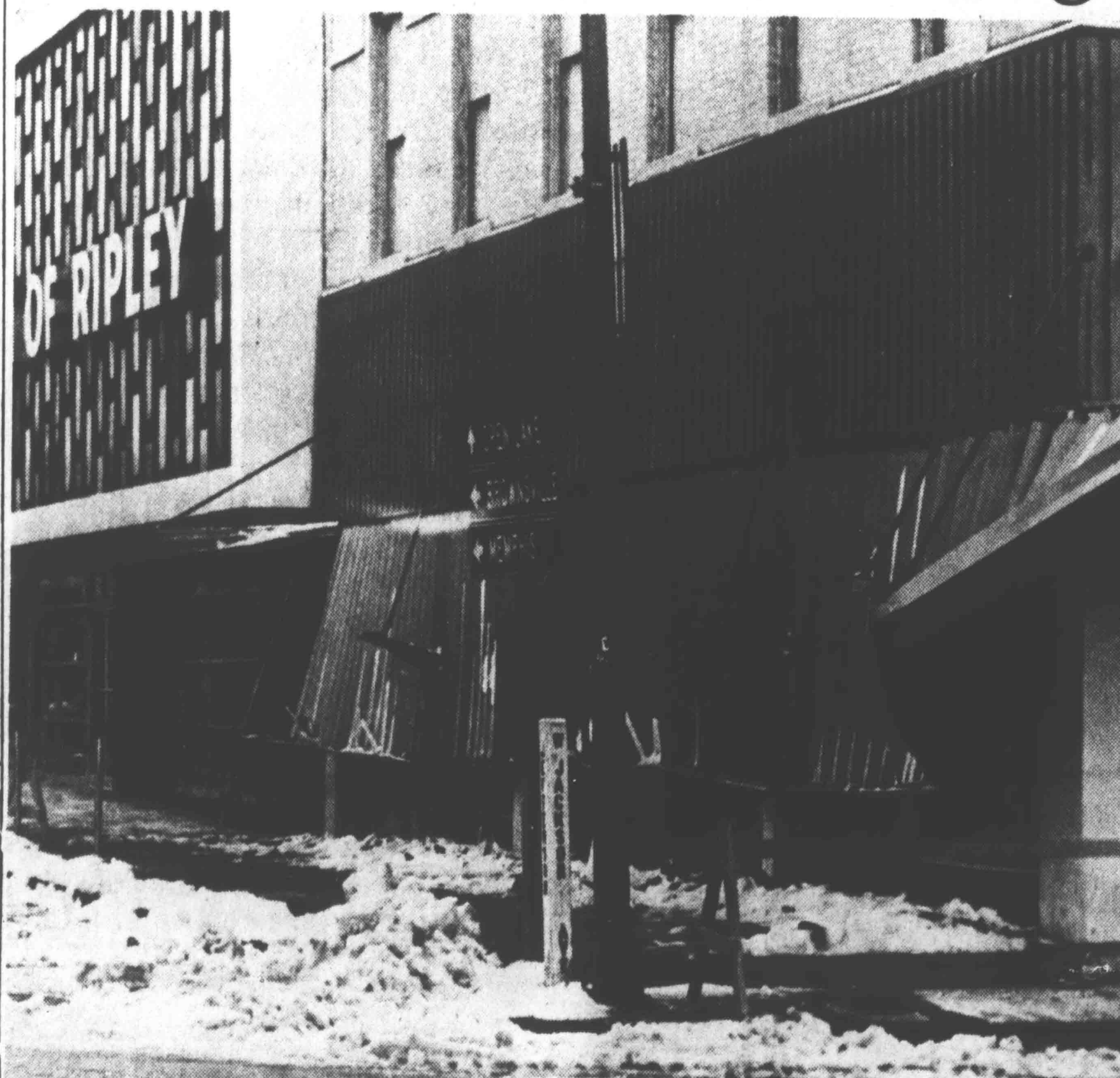
METAL AWNING FELL under the weight of snow and ice about 5:30 p.m. Monday on the former Shainberg's building in Ripley, now owned by Bank of Ripley.
